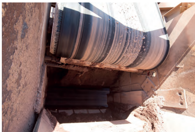
Figure 2. The lines on this belt tell a story of deficient cleaning and mistracking leading to dust, spillage, and carryback.
