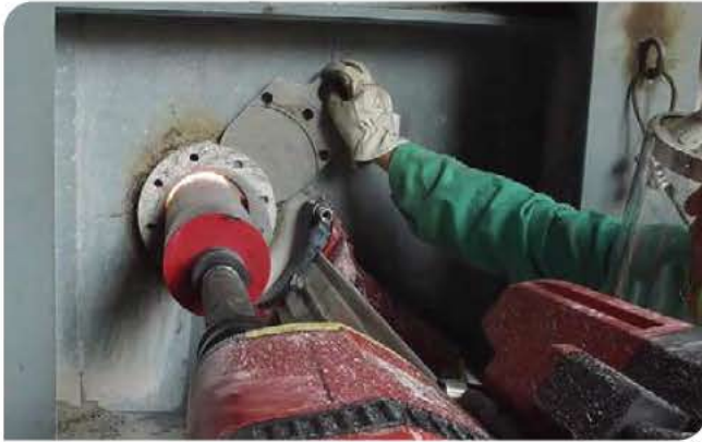
Above - Figure 3: Drilling for a new air cannon on an operating preheater by a trained specialist. ©Martin Engineering 2023.
