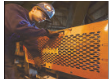
All moving or rotating components should be guarded, regardless of location.
