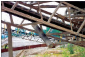
Unguarded return rollers over walkways can fall and produce a serious hazard.
