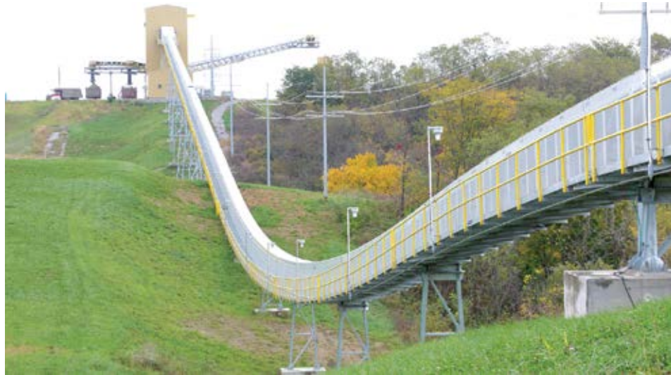
BEUMER used advanced design tools and a holistic approach to design, deliver and install a 4-mile-long, single-flight conveyor system in less than 14 months. (Photo: BEUMER)
