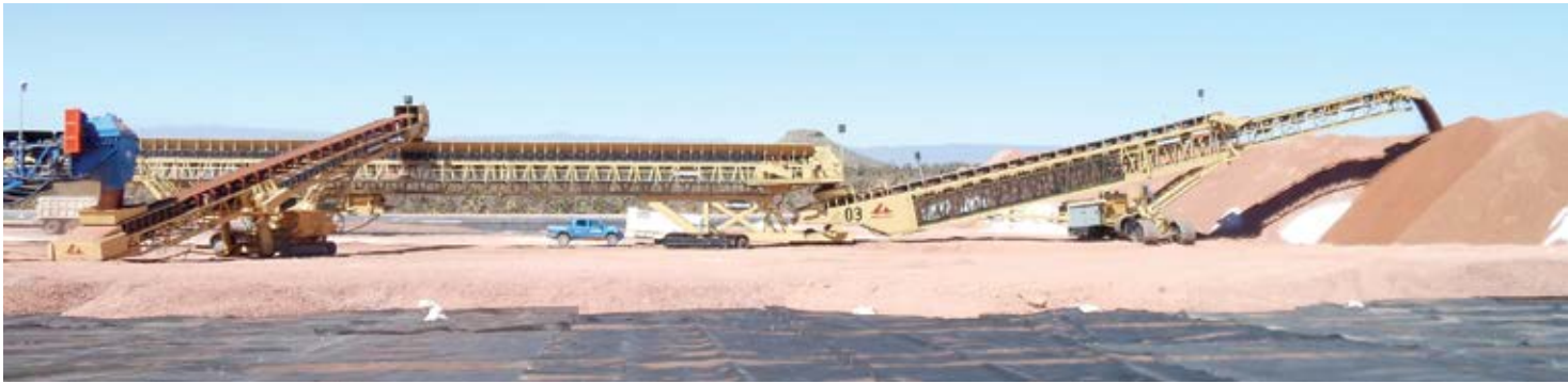
PilePro Automation and the similar heap leach automation system for the TeleStacker Conveyor were designed to be integrated into a parent control system for conveyors. Above, a conveyor system ends with a Telestacker Conveyor at a site in San Felipe, Mexico. (Photo: Superior Industries)
