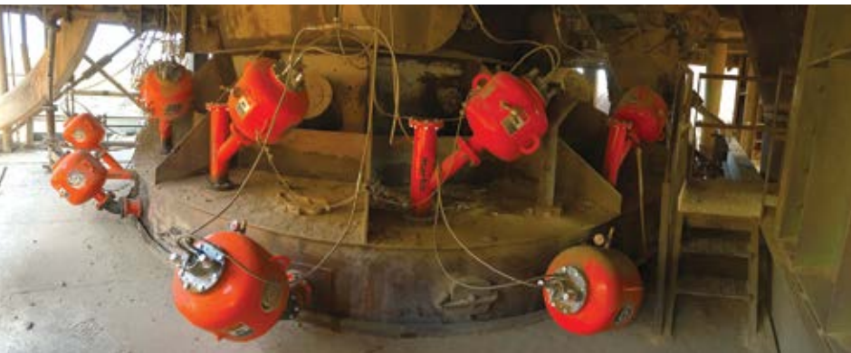
Air cannons can be useful in preventing troublesome material accumulation in process equipment, minimizing the need for downtime and manual labor.
