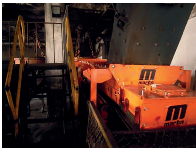
Figure 6. Installers used the Mitered chute design for #185 with a tail box, skirtboard extensions, and curtains.
