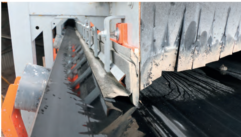
Figure 4. The proper skirtboard extensions and curtain placement drastically reduce dust emissions.
