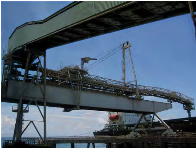
Figure 4. Belt tracking keeps loads centred and minimises dust from spillage and disruption.
