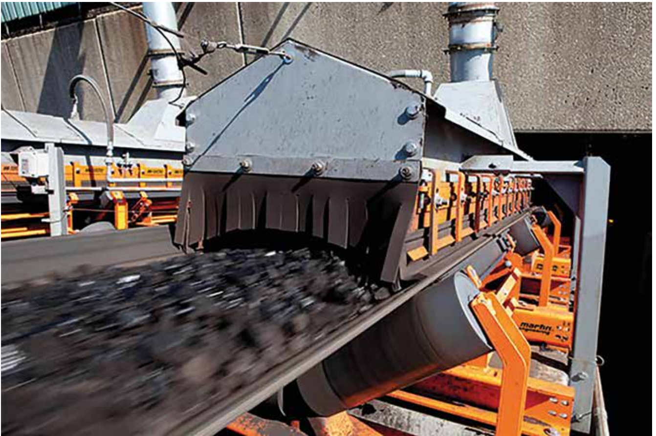
Figure 5: The reconfigured conveyor controls emissions for improved safety and easier maintenance.
