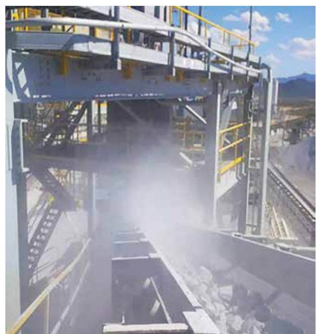
Figure 4: Bulk material drops onto a moving conveyor belt, creating dust and spillage.
