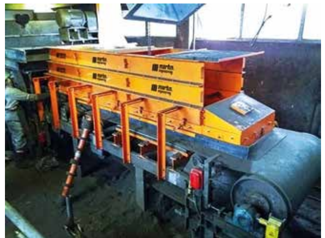
Figure 1: With the proper enclosure design, dust volumes can be lowered to below regulatory levels.
