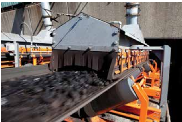
A properly configured conveyor controls emissions for improved safety and easier maintenance.
