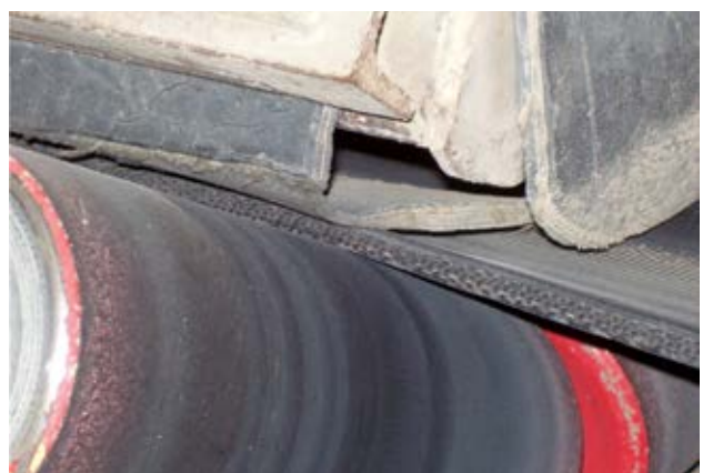
Figure 4 — Old belting used as a lay-in seal traps material between the seal and belt.
