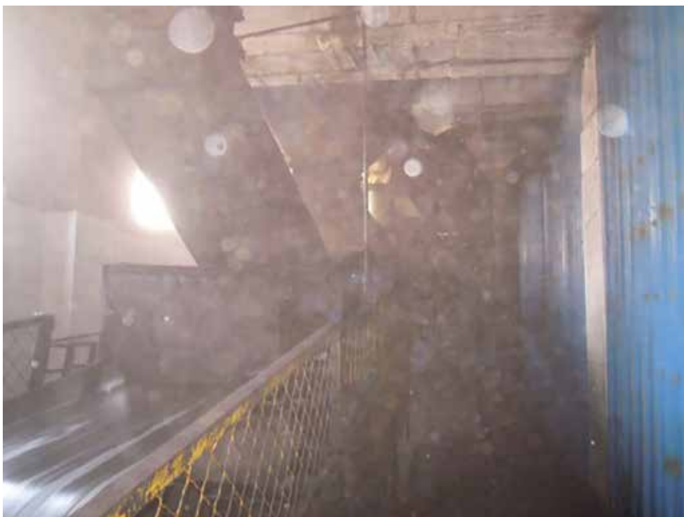
Access to the #111 transfer point was seriously limited by the lack of visibility caused by dust.
