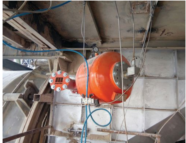
A solenoid box located far from heat and danger areas provides easy access.
