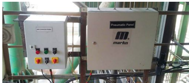
The outward facing valve allows safe servicing by one worker, without a shutdown.
