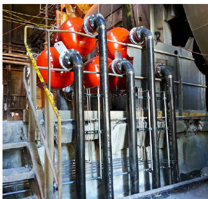
4.5-in. (11.5-mm) pipes lead down to holes drilled into the concrete floor, then continue under the subfloor.
