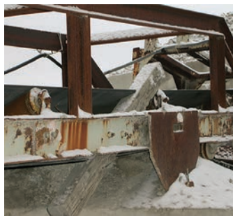
Attempt to control critical mis-tracking symptoms using a timber.
