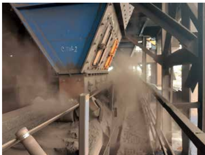
Dust accumulation on rolling components can cause abrasive damage and premature failure
