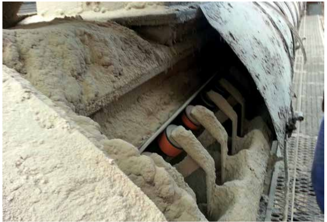
Access for replacing rolling components is a serious concern for dusty applications
