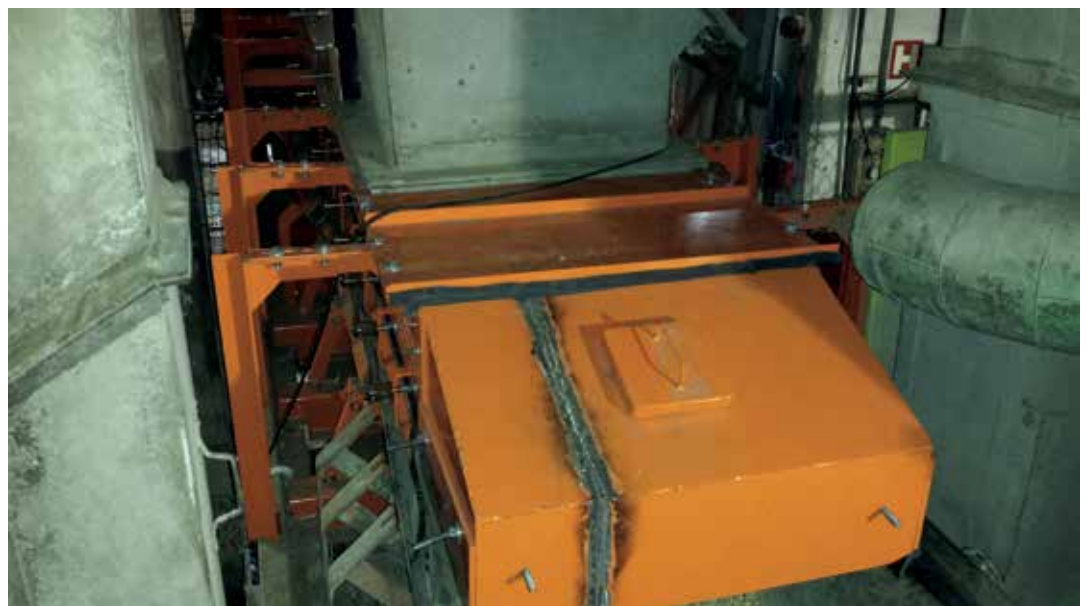
Accessible inspection doors help workers safely identify problems early
