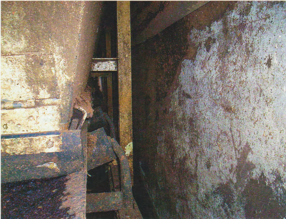
10 This conveyor was positioned so close to a tunnel wall that service and upgrades are extremely difficult
