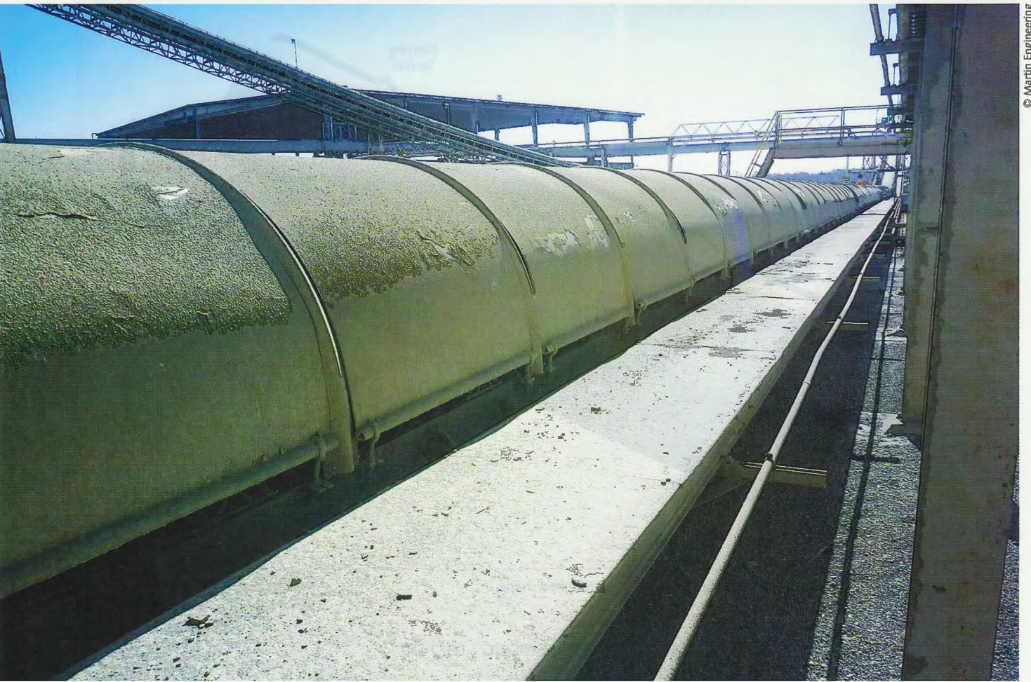
5 This cable tray blocks access for efficiently replacing idlers
