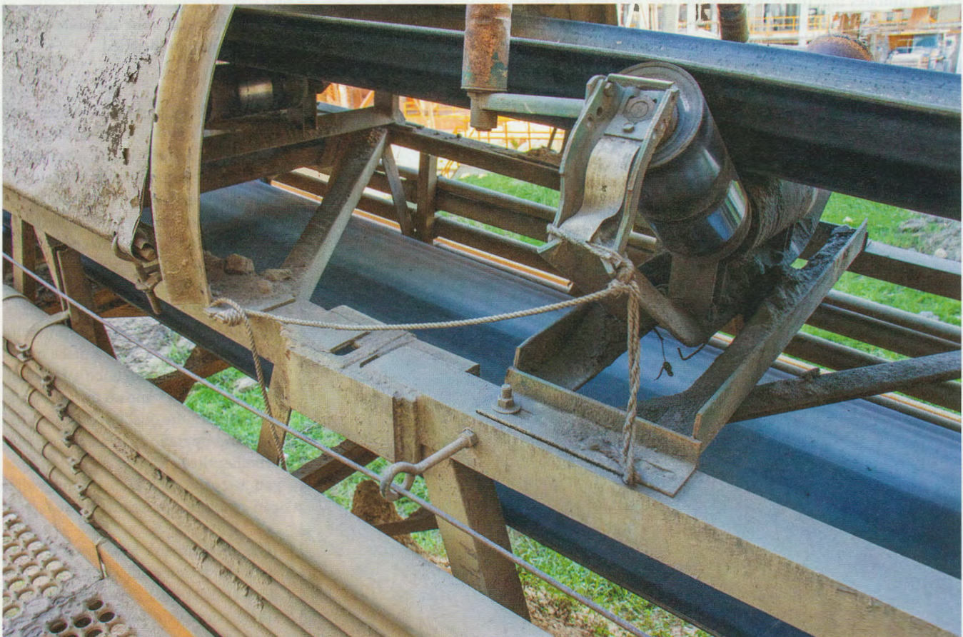
5 Most belt tracking issues result from misalignment of the structure, pulleys and idlers
