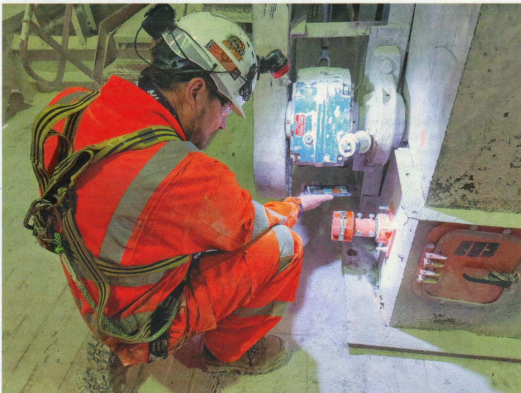
5 Aaron Bartram of Martin Engineering uses the Martin Mobile App to calibrate one of the newly-installed N2® conveyor belt cleaner smart monitoring devices
