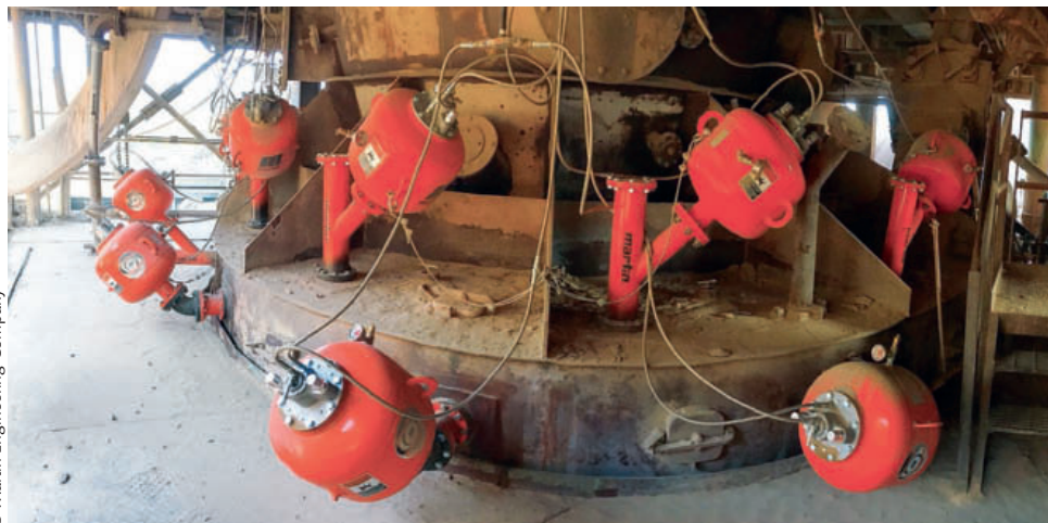
5 Air cannons can help prevent accumulation, while minimizing the need for downtime and manual labor
