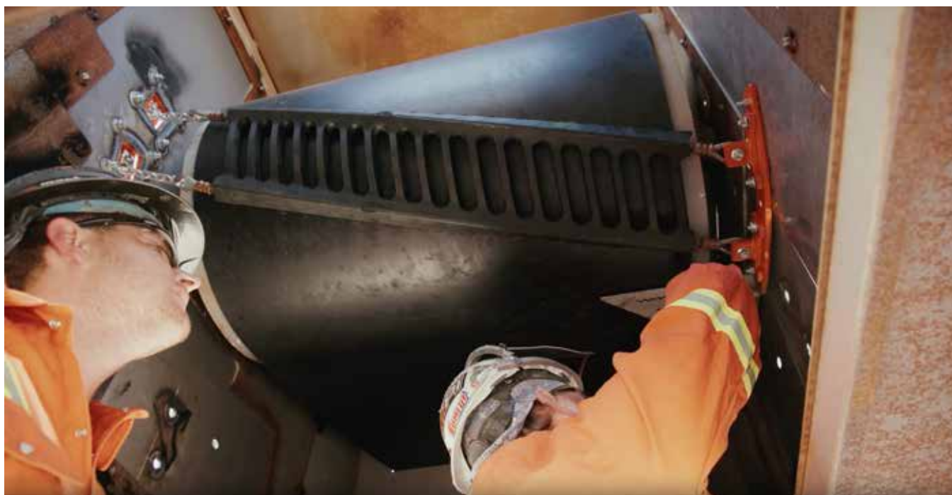
© Martin Engineering Company
