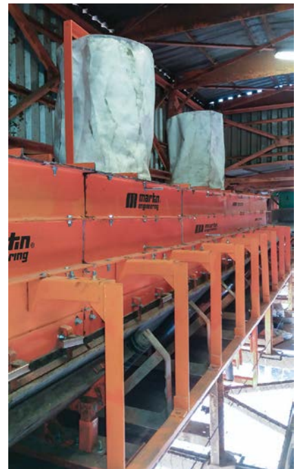
The new loading zone featured a sealing system that mitigated spillage and dust supported by dust bags.
