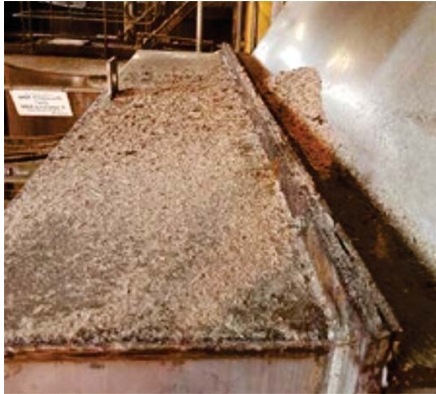
Fine dust and shards of wood spilled along the belt path and piled on surfaces.
