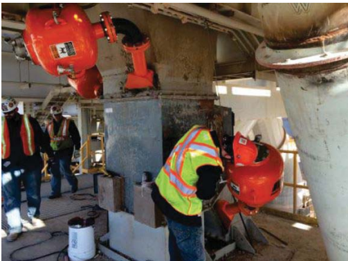
Mounted down three levels of the chute, workers have good access to the cannons for easy maintenance.
