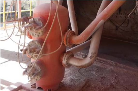
The workers at a cement plant in Panama were running out of space around their preheater.
