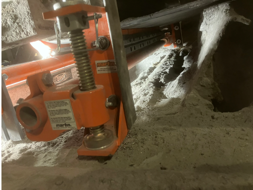
Installation of Martin QC1™ HD to improve fugitive material under the belt.
