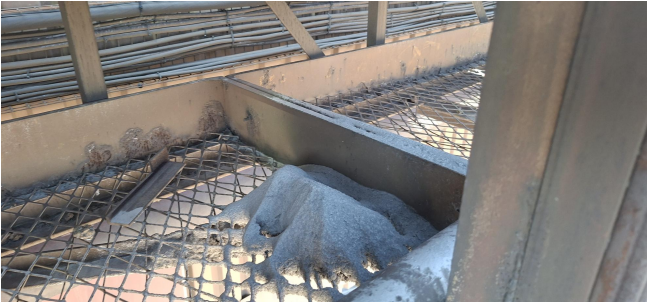
Spillage due to ineffective belt cleaning causing safety hazards
