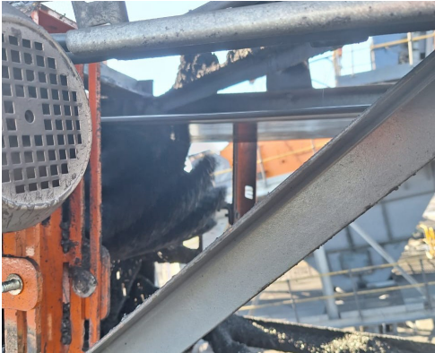
Unsafe, time consuming Brush Cleaner maintenance with restricted one-sided walkway access
