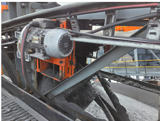
The customised bracket now allows quick, simple access, making maintenance safer and more efficient.
