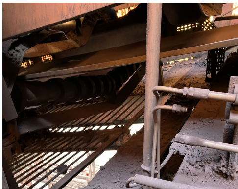
Elimination of material loss underneath the belt
