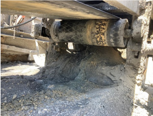
Poor belt cleaner performance was resulting in carryback, spillage and excessive maintenance.
