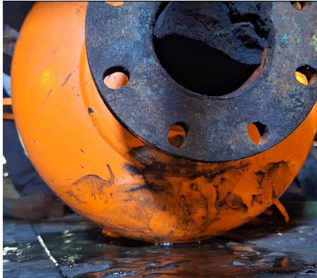
Old Air Cannon has been removed and damaged due to lack of maintenance
