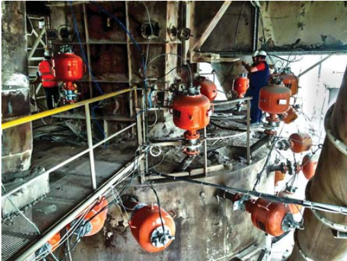
29 Martin® Hurricane Air Cannons, each with a 70 liter reservoir, were installed in strategic locations.
