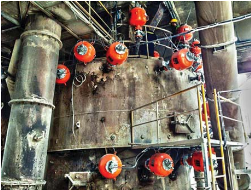
Installed in a series and sequenced for maximum effect, the air cannon network can be timed to suit specific conditions.
