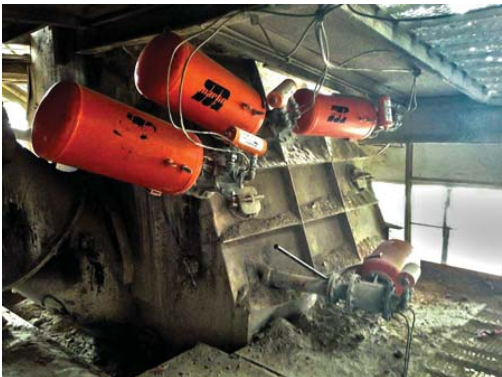
22 existing Tornado Air Cannons were upgraded with a Martin® Piston Return Reservoir to reduce operating costs.
