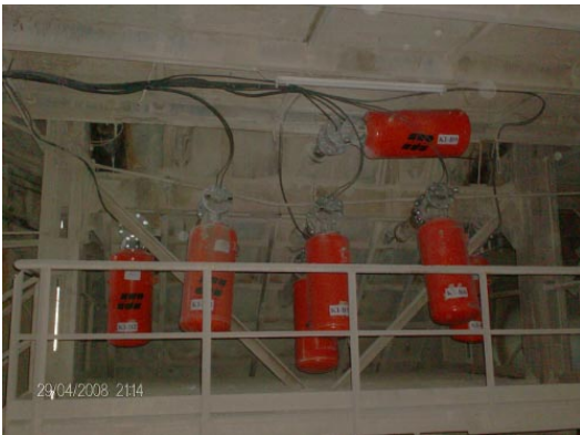
Technicians from Martin Engineering Turkey installed a battery of 31 Martin® Air Cannons
