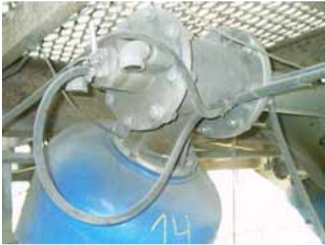
Installed at the Matozinhos plant, the Martin® XHV Air Cannons with Martin® Tornado Exhaust Valves provide more output force to improve material flow.
