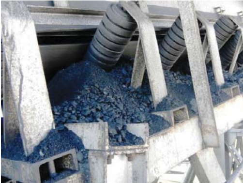
A coal-fired power plant in Turkey was having trouble with dust and spillage at a conveyor transfer loading point.
