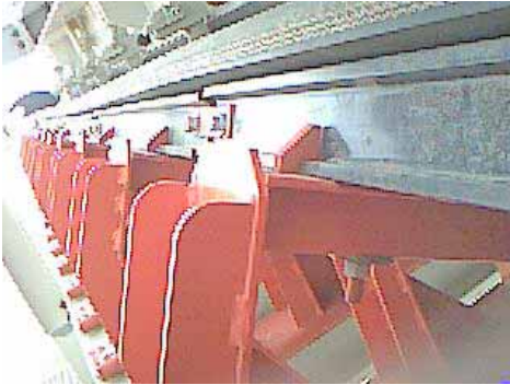
New conveyors at a Peruvian gold mine include modular, slide-in cradles to support the belt.
