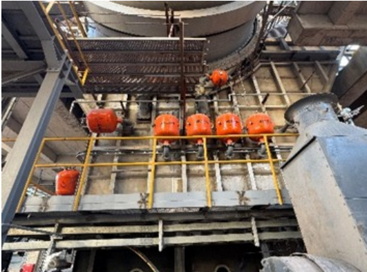
At integrated cement plants, efficient upstream material handling and pyroprocessing material flow is critical.
