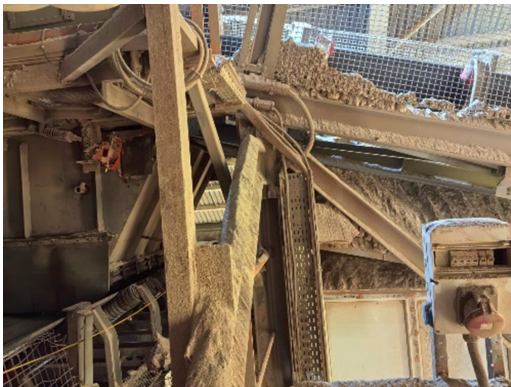
The previous arrangement caused serious carryback accumulation along the conveyor's return path.
