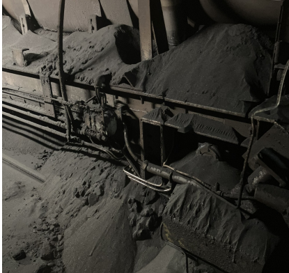
Material loss causing safety hazards and production loss
