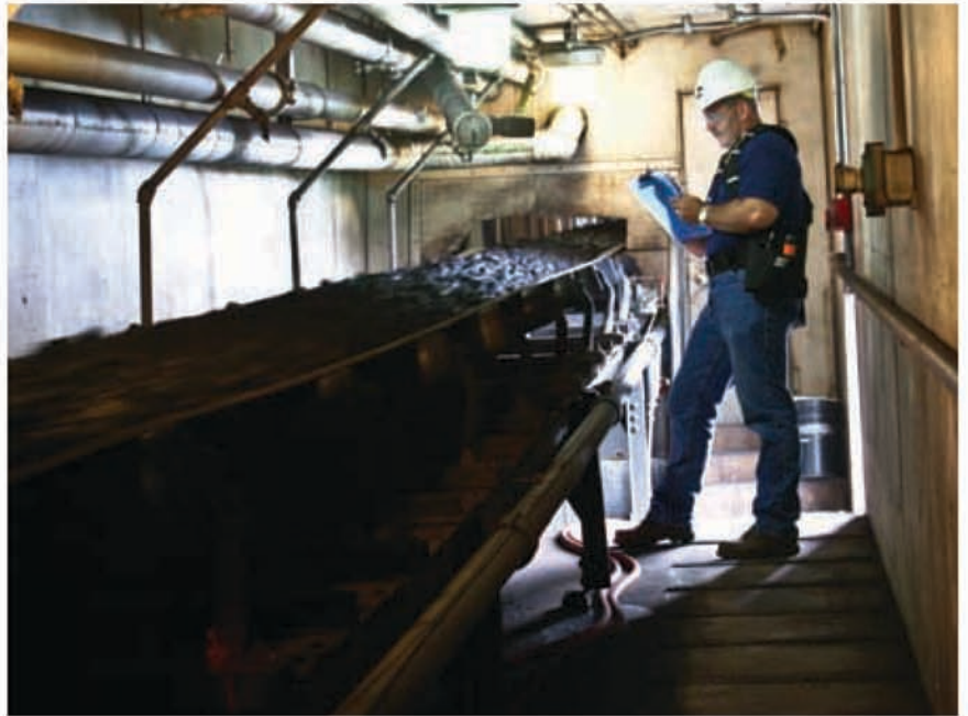
In the best operations, maintenance workers routinely “walk” the conveyor system looking for indications of potential trouble.
