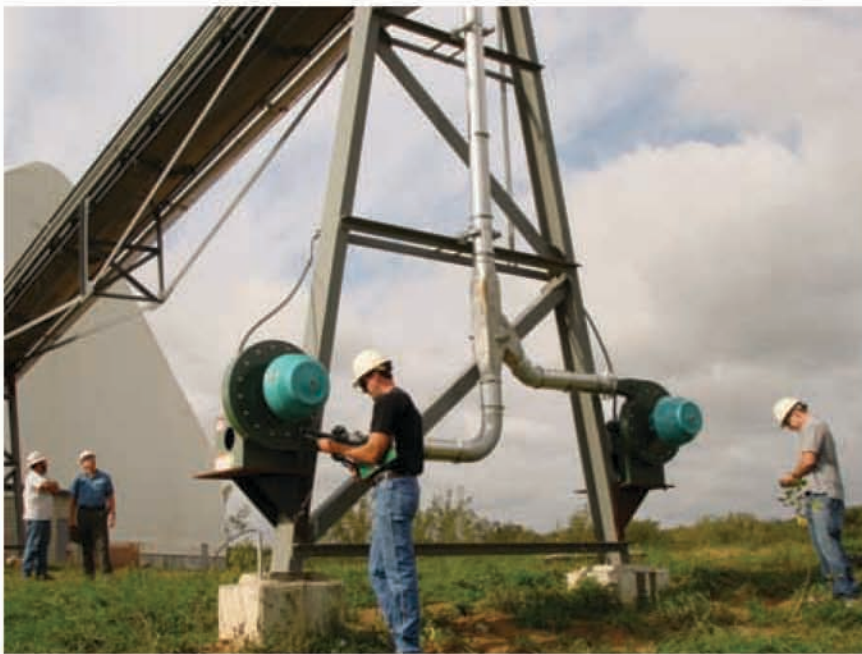
Conveyor maintenance provides timely intervention to keep performance levels at plant standards and avoid unscheduled production-crippling outages.
