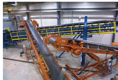
At Martin Engineering's Center for Innovation, the process simulation area incorporates a three-belt recirculating conveyor loop for observation of material flow and component life.
