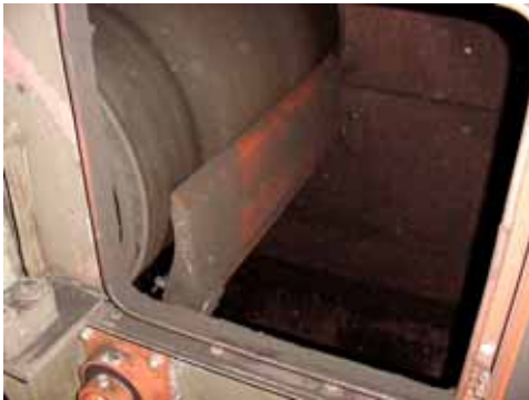
Martin® QC1™ Cleaner XHD installed at Neal Station South.
