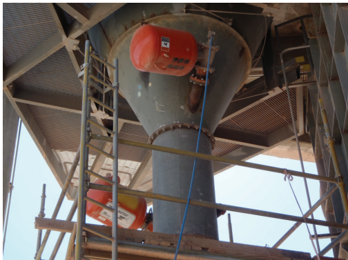
Several of the cannons were located in the entry to the kiln, cooler inlet and the preheater tower.
