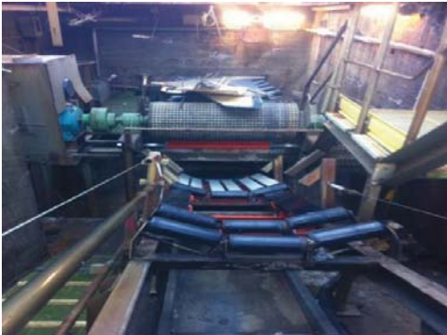
Martin provided several solutions to eliminate the carryback, and used air cannons to improve the flow of material.
