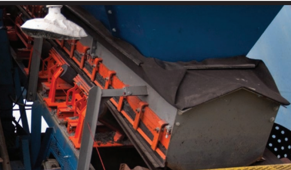
Components of the new conveyor architecture are incorporated in the loading zone of the shiploader conveyor at the coal terminal at Port of Seward, Alaska.
