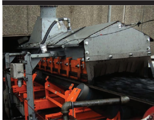
The enlarged settling zone on this transfer point at the Kansas power plant allows dust to settle out of the air.
