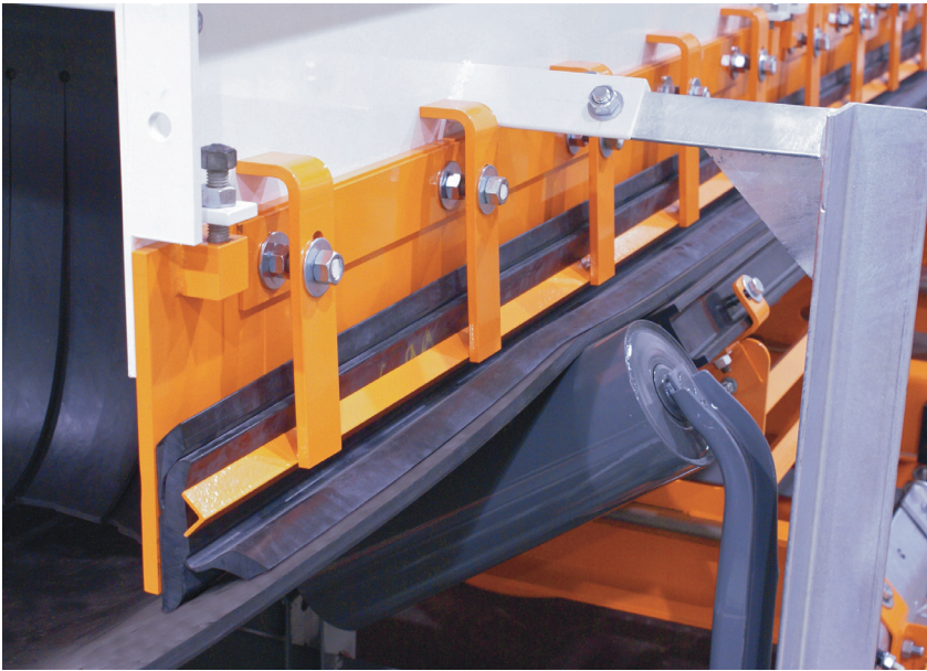
Skirtboards help reduce spillage and dust, containing the load until it assumes a stable profile.
