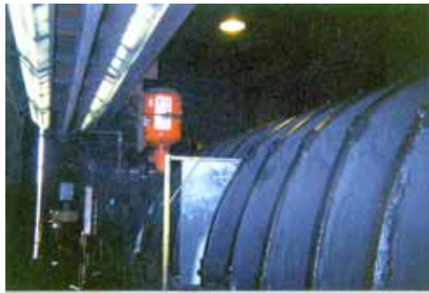
A Martin® Air Cannon is installed on each vacuum filter at Ispat Inland's taconite processing plant.
