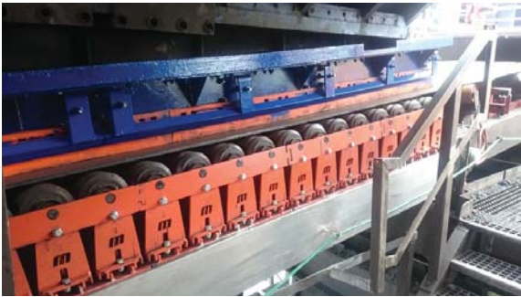
Martin Technicians installed seven Martin® High Speed Impact Cradles along the length of the module 3 feeder unit.
