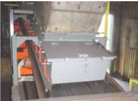
A Martin® Tail Sealing Box with Martin® Steel Inspection Door was installed to prevent material from spilling out the back of the loading zone.
