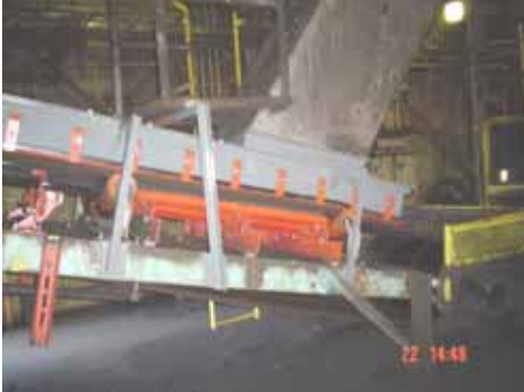
A Martin® Light Duty Impact Cradle was installed under the loading zone of Conveyor #9.
