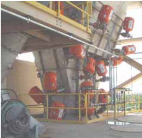
Installation of the air cannon system was performed by MartinPLUS® Installation Services.
